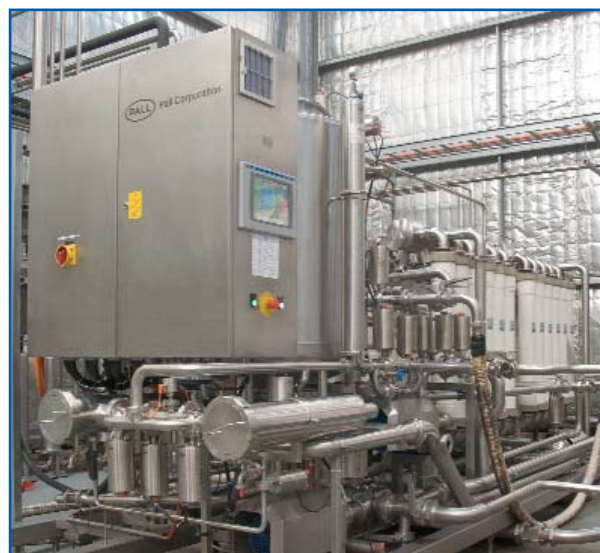
Oenoflow HS-24A System at Yalumba
